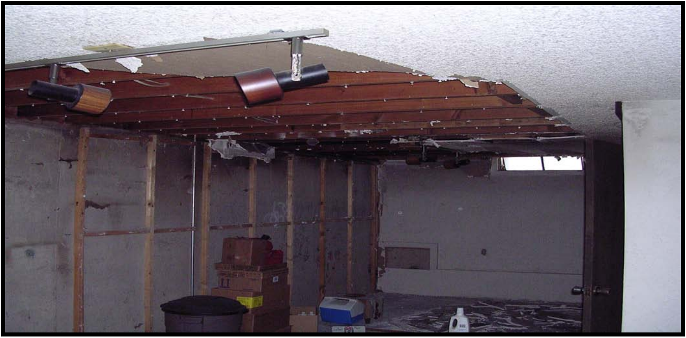
Unit 3 Debris Removal by Owner Based on State Farm's False Coverage Representation PAC Photo May 16, 2007 Wall material later proved to be asbestos containing.
